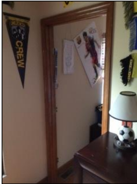
33. Missing Door Slab & Hardware
