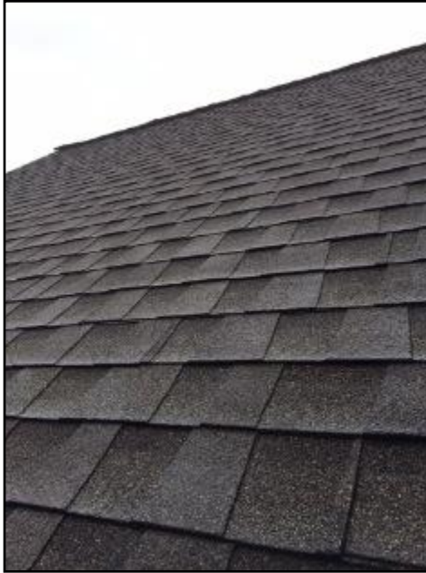
1. Wet roof surface hides flaws
