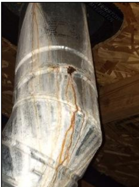
30. Rust, dirty, obstructed
