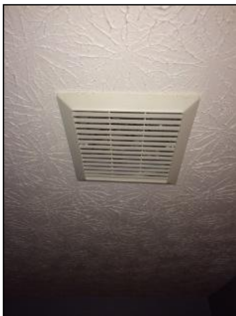
36. Not Vent to Exterior- The bathroom fan vent...
