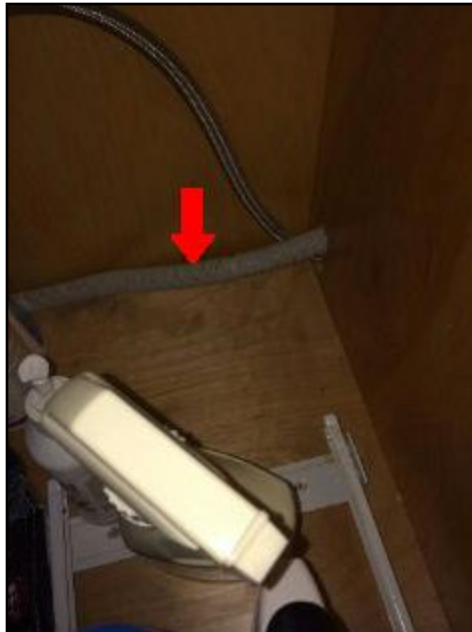
38. Backflow prevention missing
