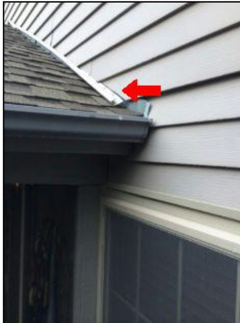
2. Siding Damage: Siding has minor damage. An...
