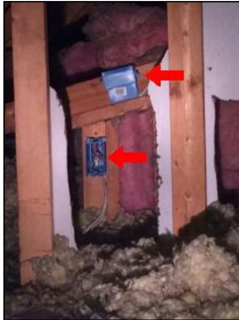
15. Cover loose or missing
