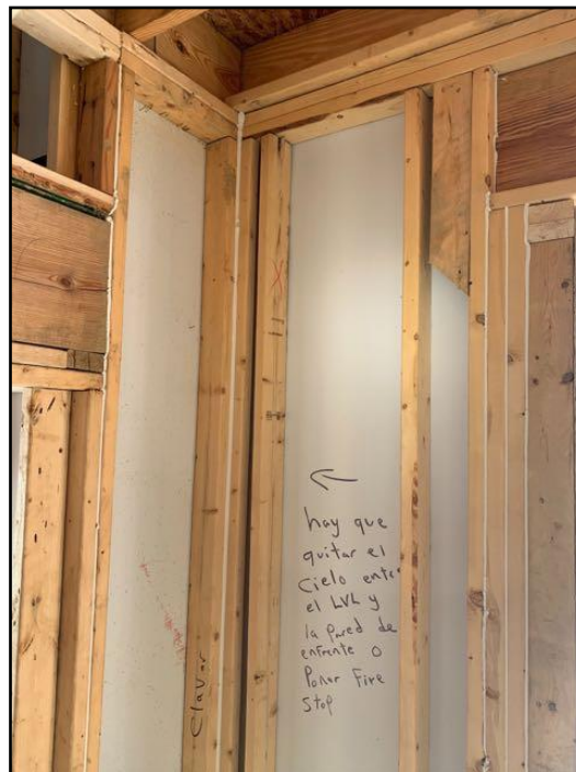
53. The use of damaged or poor quality framing...
