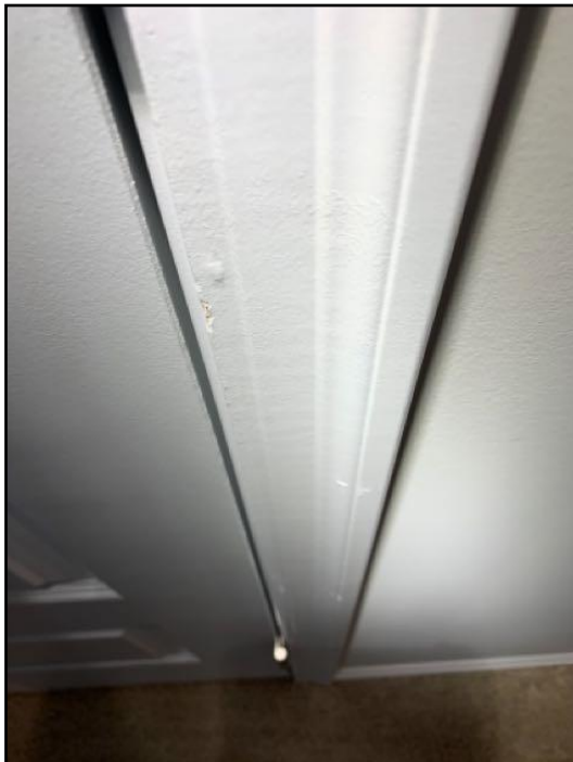
111. The door slab has cosmetic defects in the...
