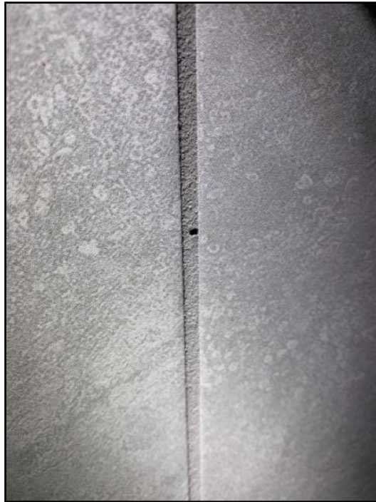
100. Grout loose, missing or deteriorated
