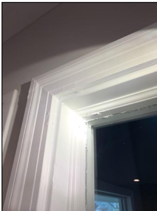
116. Low-quality paint work was observed trash i...
