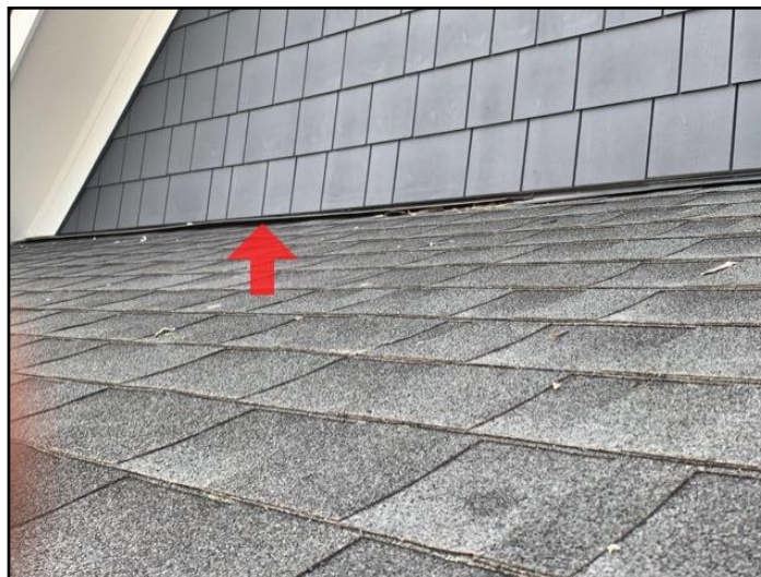
2. Damage, loose, open seams, patched
