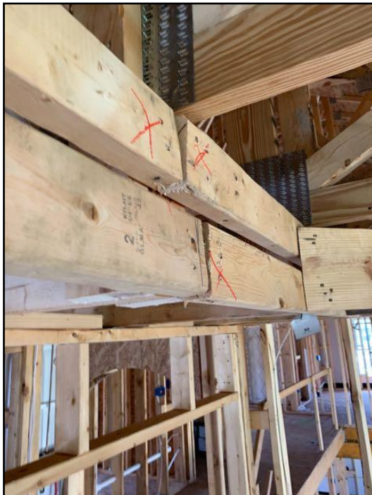
49. The use of damaged or poor quality framing...
