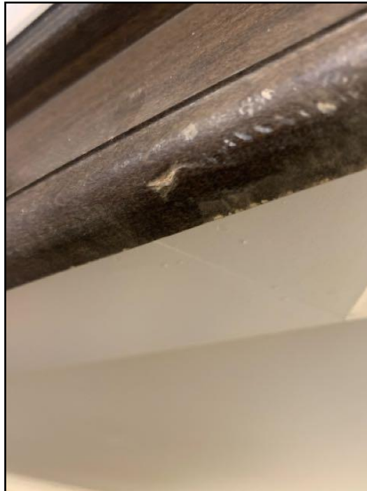
121. The finish has imperfection, unfilled voids...
