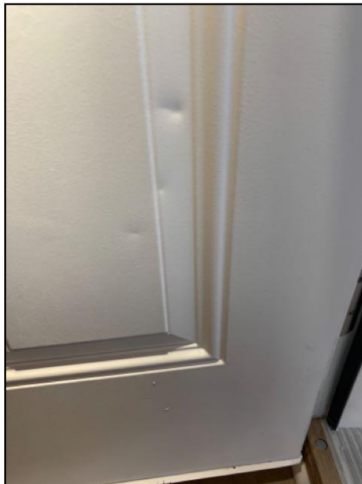
115. The door slab has cosmetic defects in the...
