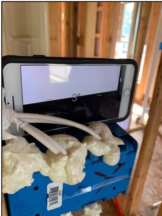
45. Leaning, bowing, buckling
