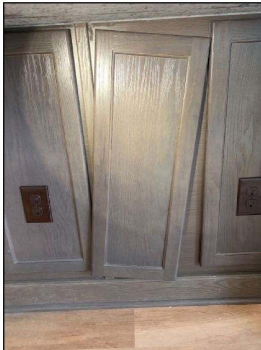
117. Pieces missing or loose
