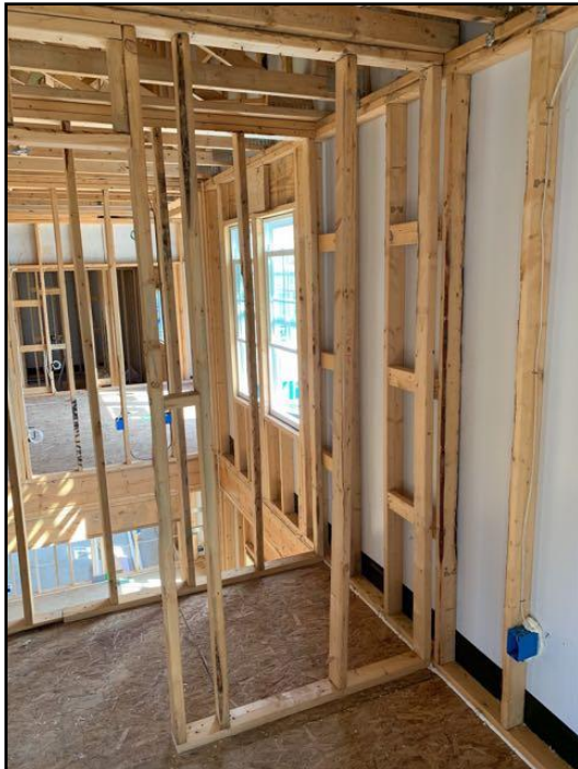
47. Leaning, bowing, buckling
