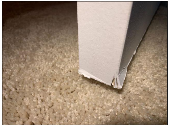
112. The door slab has cosmetic defects in the...
