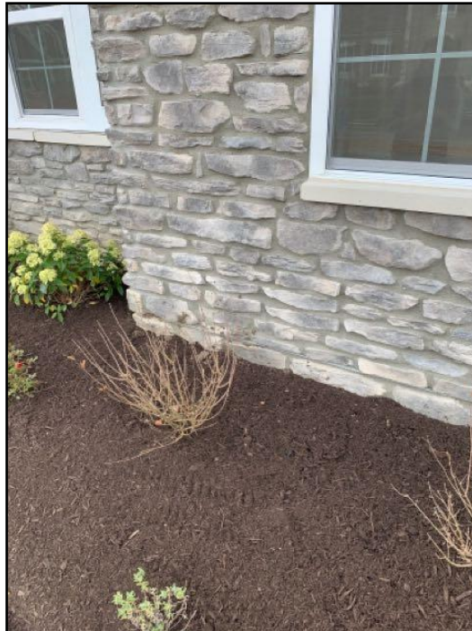
11. Missing, ineffective weep holes or flashings
