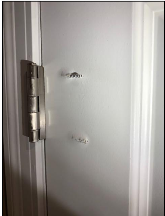
114. The door slab has cosmetic defects in the...
