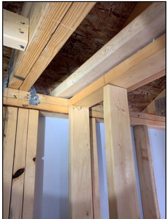
50. The use of damaged or poor quality framing...
