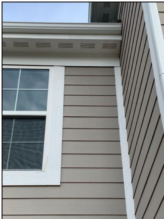
6. The exterior trim has cosmetic defects in...
