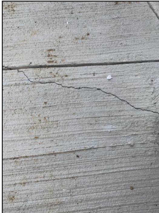
25. Cracked or damaged surfaces
