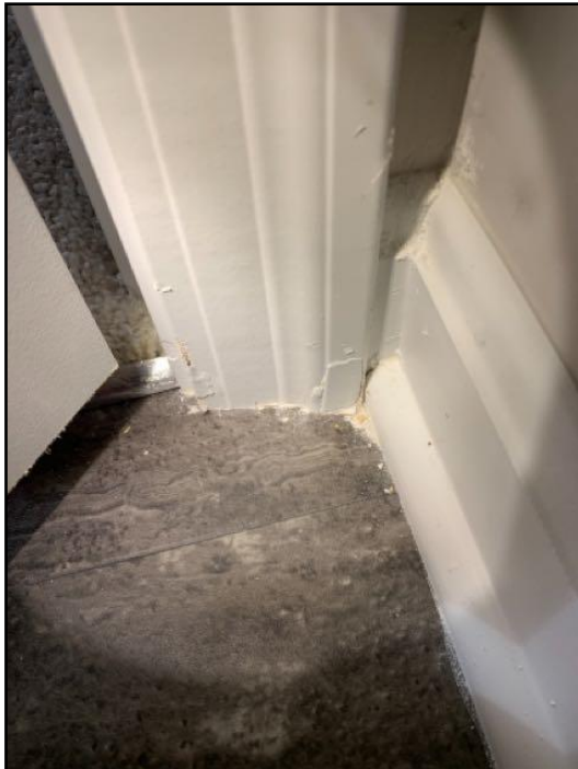
113. The door slab has cosmetic defects in the...
