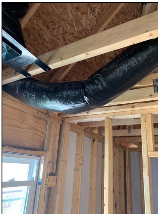
81. The support strap appear to be missing,...
