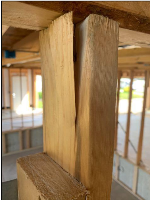
51. The use of damaged or poor quality framing...
