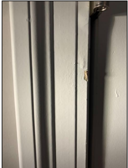
110. The door slab has cosmetic defects in the...
