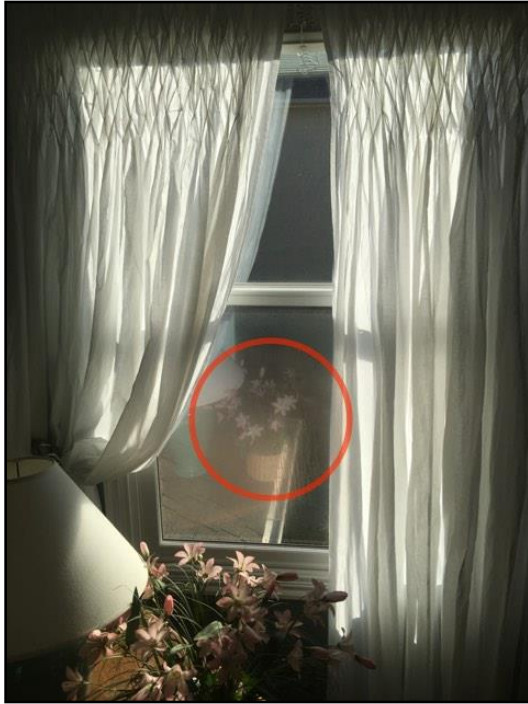
27. Fogging or other moisture between the panes...
