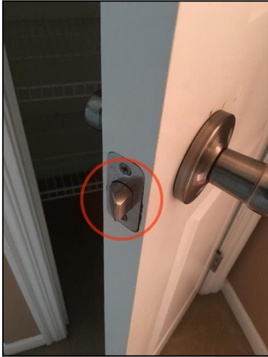
32. Does not latch properly
